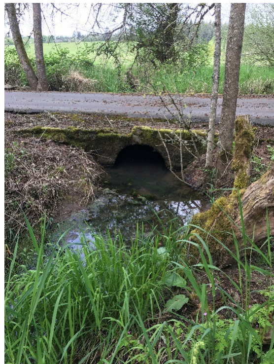
Figure 3-4 | Private road crossing and channel incision (45.438127, -122.879317)
